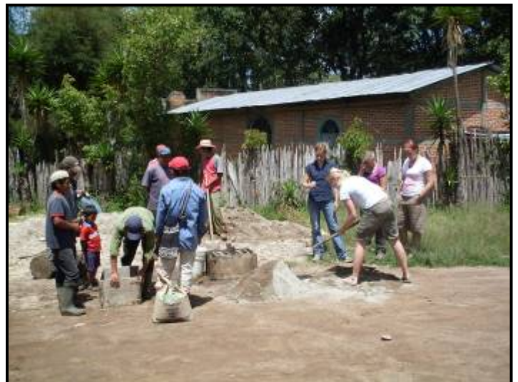
Villagers and Help International volunteers, working in the construction of grease trap box for the gray water filters.
